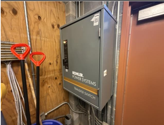
25 - AUTOMATIC TRANSFER SWITCH
