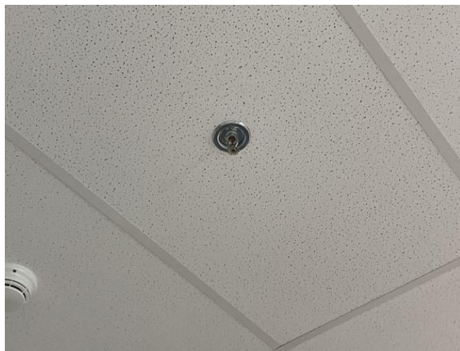
28 - FIRE SUPPRESSION SYSTEM
