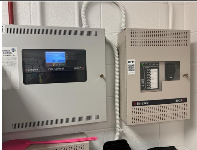
26 - FIRE ALARM PANEL / INTERCOM/PA SYSTEM
