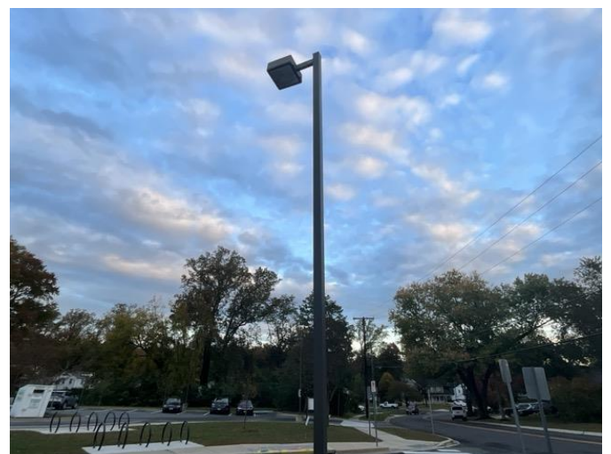
36 - POLE LIGHT FIXTURES
