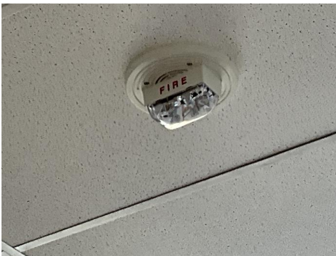
27 - FIRE ALARM SYSTEM
